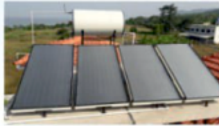
Solar Hot Water System
